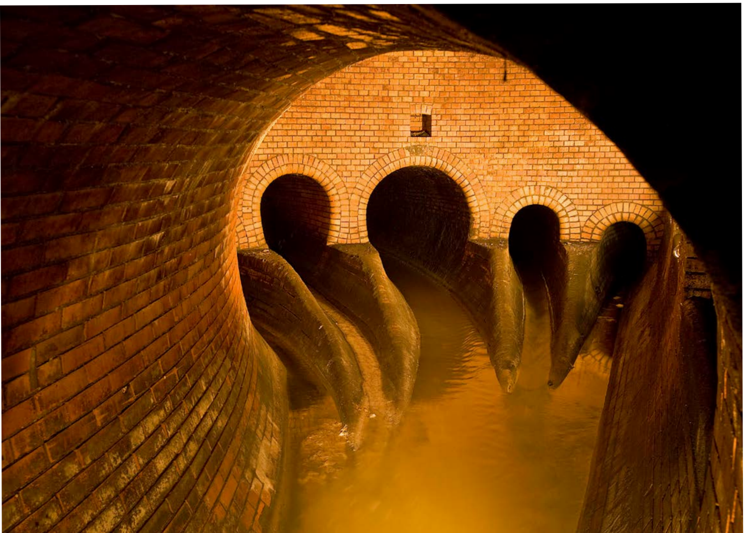
Photo 25: The way of the waste water
