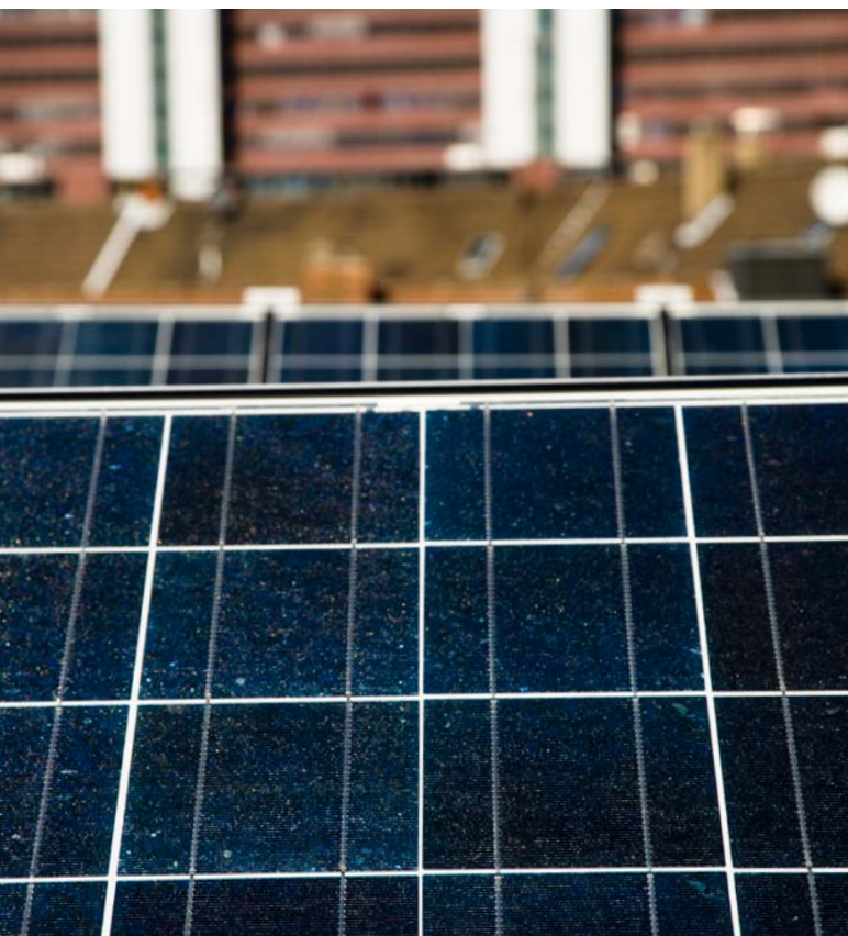
Photo 26: Example image - solar panels on the roof
